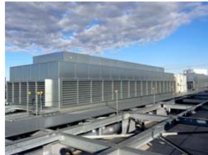
Outdoor air-conditioning equipment: modular chillers on the roof
