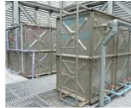
Surrounding water tanks with shade mesh protects them from direct sunlight.
