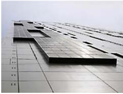
Solar panels installed at Tokyo No. 5 Data Center
