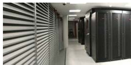
Air-conditioning system that blows cool air from walls
