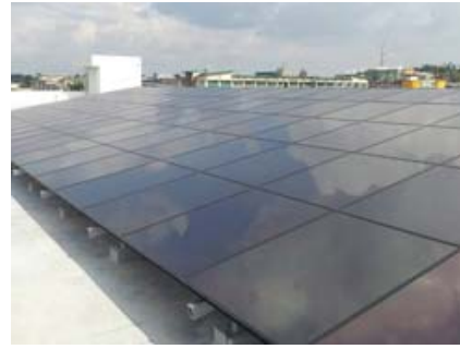
Solar panels installed on the rooftop of the Data Center building in Malaysia
