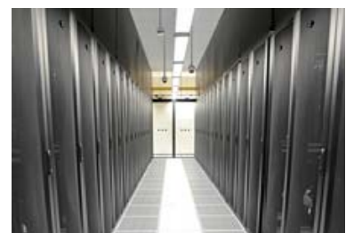
High cooling-efficiency server room
