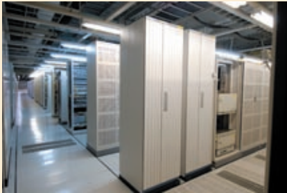
■ Equipment racks in a communications equipment room
