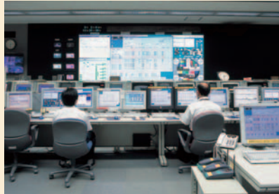
Operation room of the Tokyo Television Center
